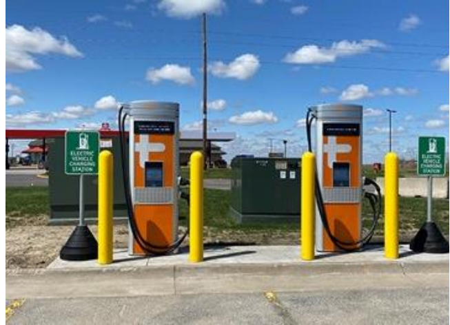
Figure 12. Example EV charging stations
